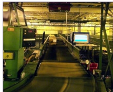
Operator Station on Conveyor System
